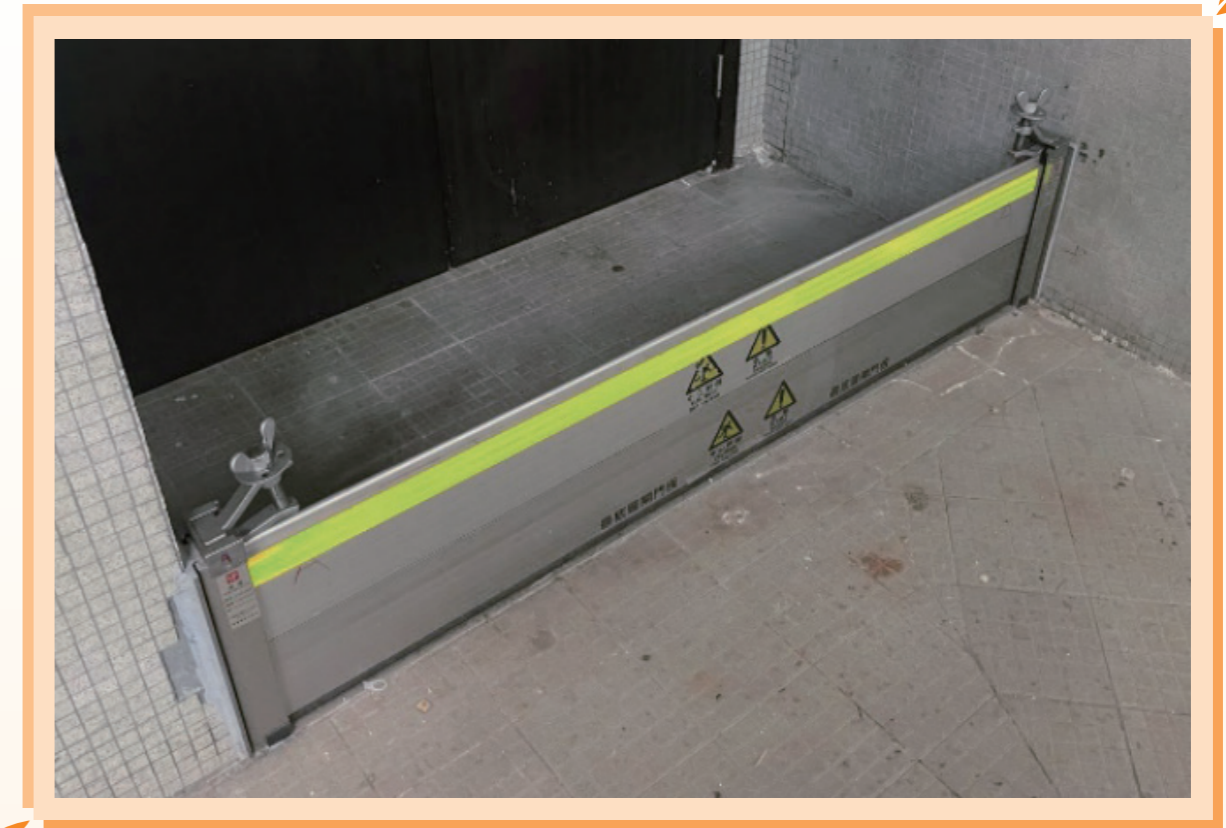
Flood Gate at Regal Airport Hotel
